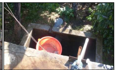
Pic. 26. Recirculation tank
