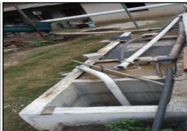
Pic. 19. Recirculation tank
